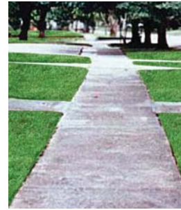
Before and After Picture of a sidewalk. Pictures courtesy of CRC of Texas-Houston (CRA associate).
